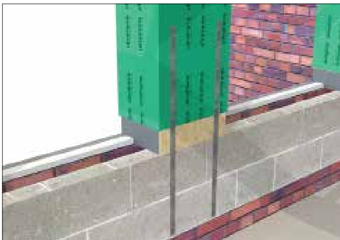
INLINE Fasten straps down inside of wall of inline column. Use suitable fixing.
