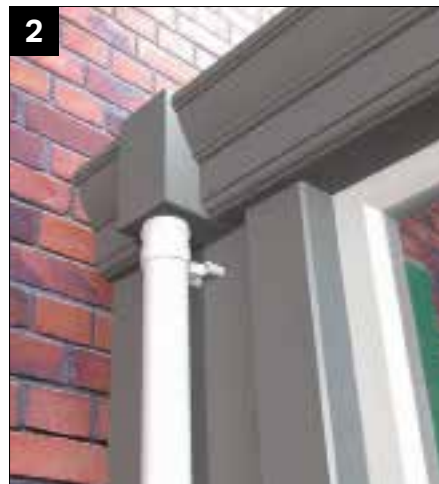
2 Elephants Trunk outlet. If it is not possible to have full height columns i.e. on dwarf wall.
