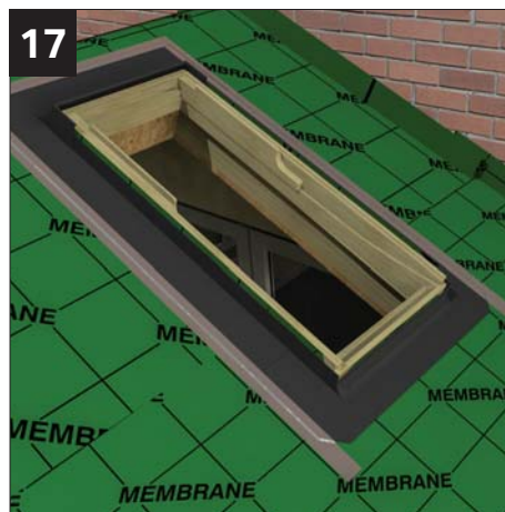
17 Apply the supplied aluminium backed butyl tape. Fit the SIDES first followed by the top to ensure a good seal.
