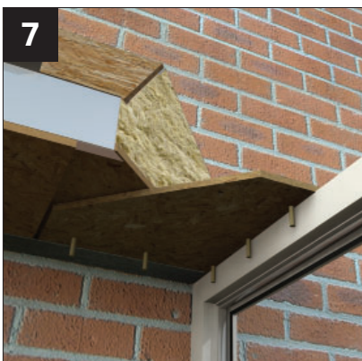
7 Ensure support shelf locates in the cut-out on the underside of the box beam
