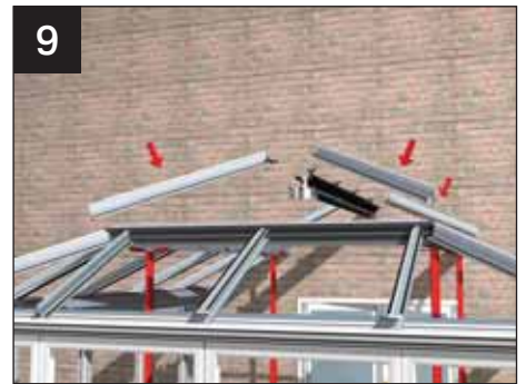
9 Using the roof location plan, build the upper roof as per section 4 of this guide.
