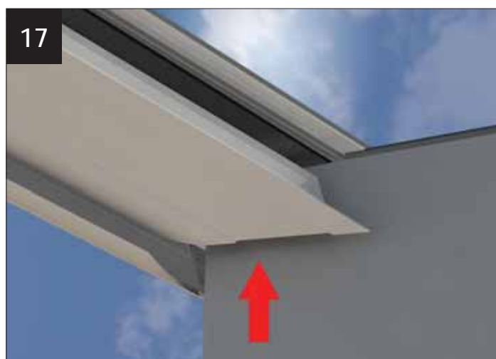
17 Classic Plus Valley cladding being fitted against internal insulated pelmet. After plasterboard and skim.
